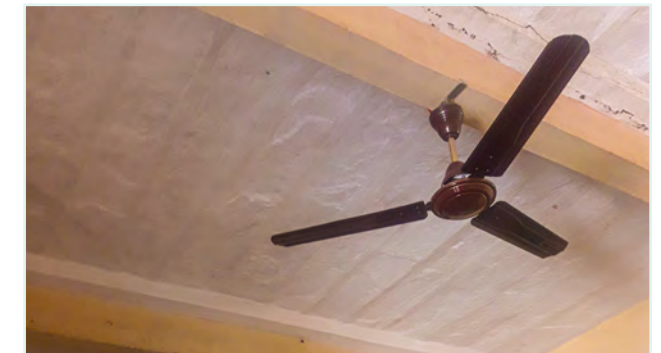
Electrical appliances running on solar power
