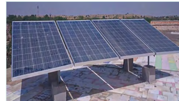
Solar panel mounted in Adarsh schools
